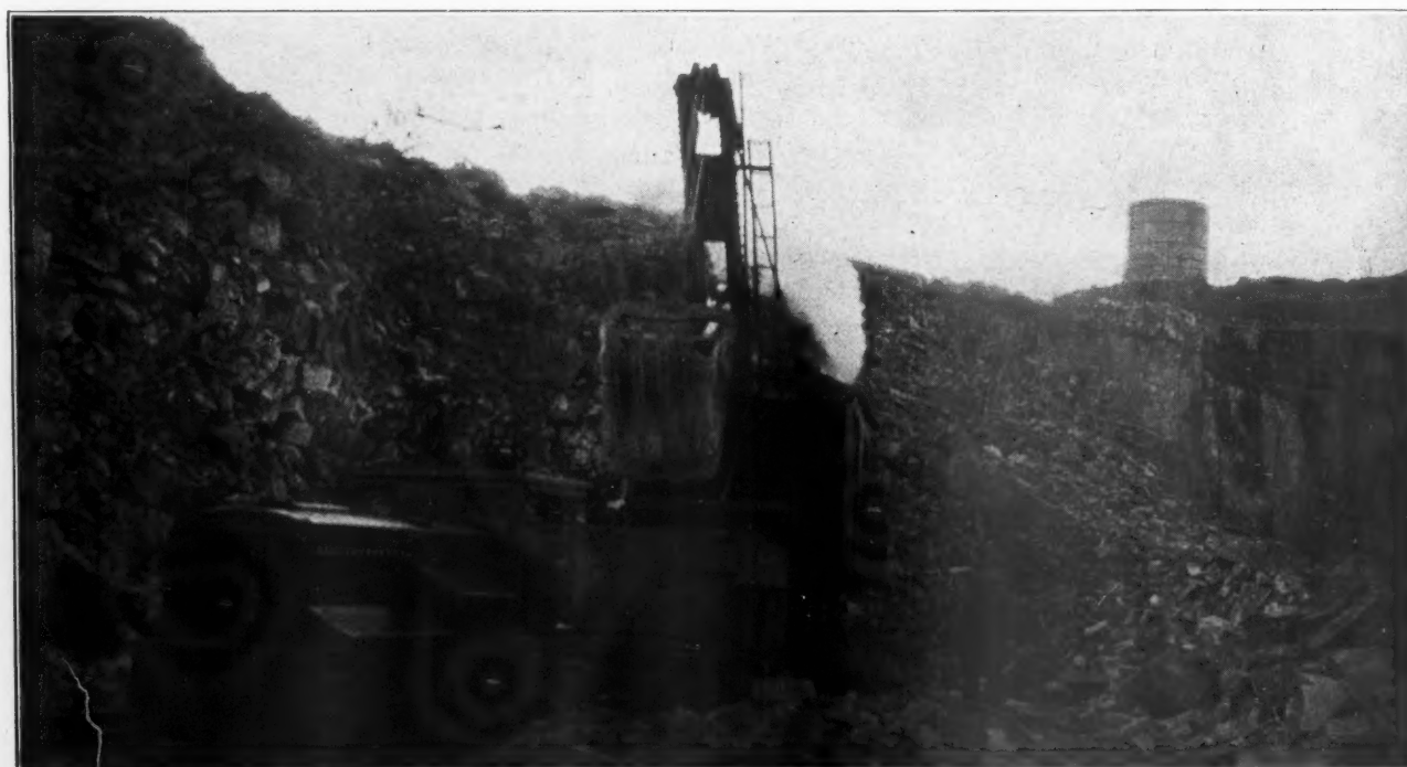
Shovels Loading Cars Drawn by Gasoline Engine at the Old Upper Level of the Quarry
